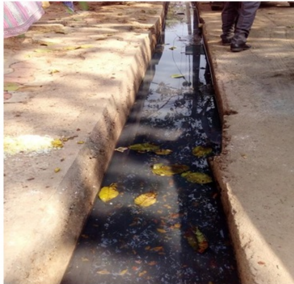
Figure 4 Drain outside the hospital with mosquitoes breeding
